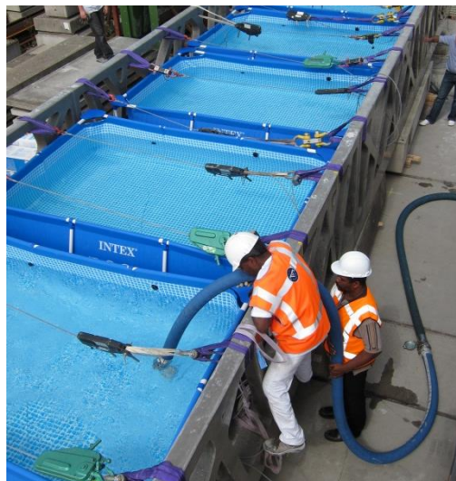
Figure 9: For the testing of the bridge, water containers were filled with water
